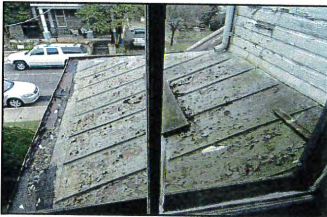
ROOF & SIDING DAMAGE
