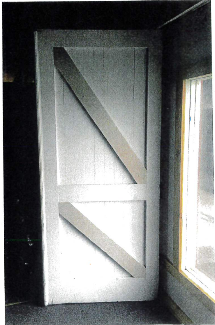
212 N. Union St. west facing doors to be restored
