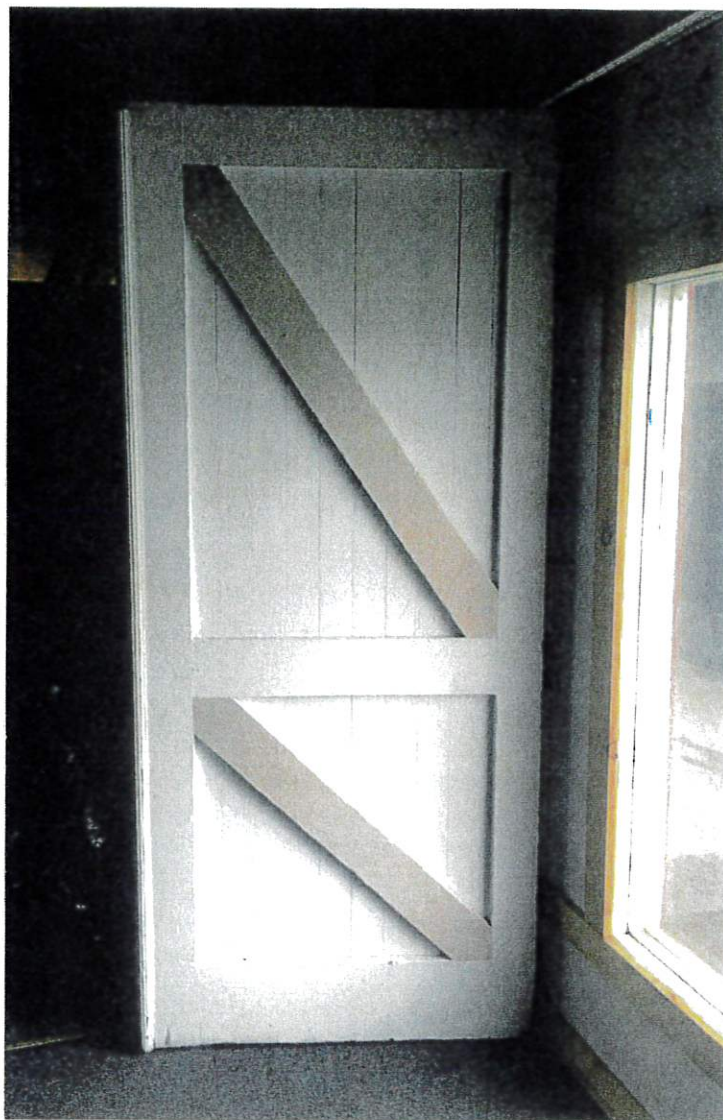
212 N. Union St. west facing doors to be restored
