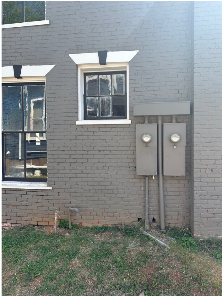
Existing electric services
