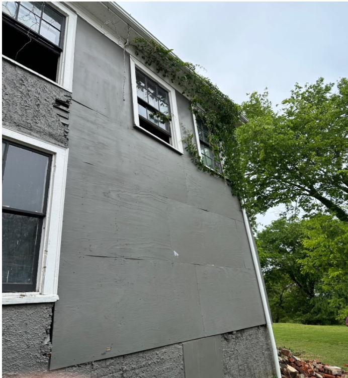
Area on East face of the façade in need of repair
