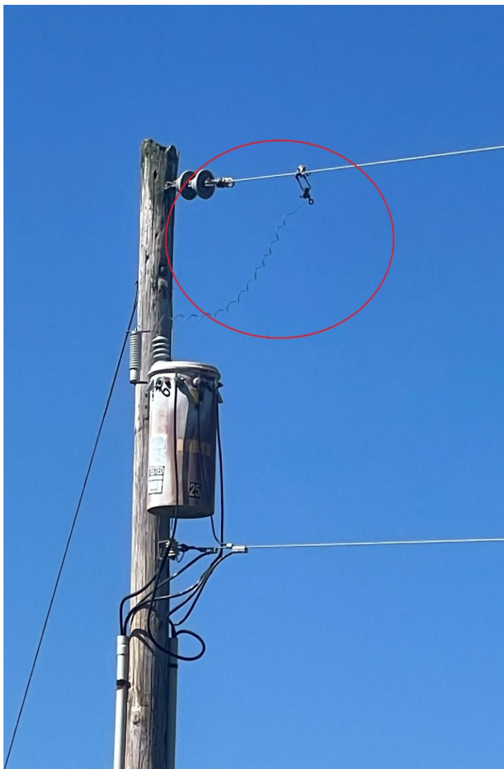
No Transformer Protection
