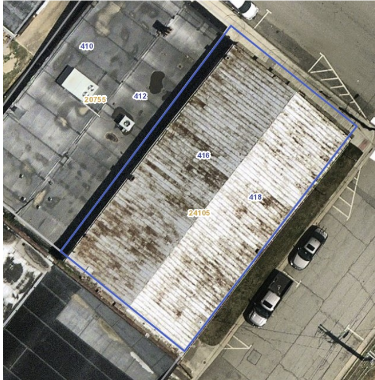
Aerial Map (Note Condition of Roof)
