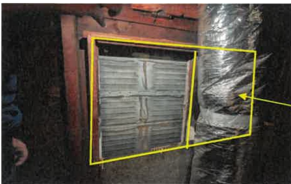
Window casing window obscured
