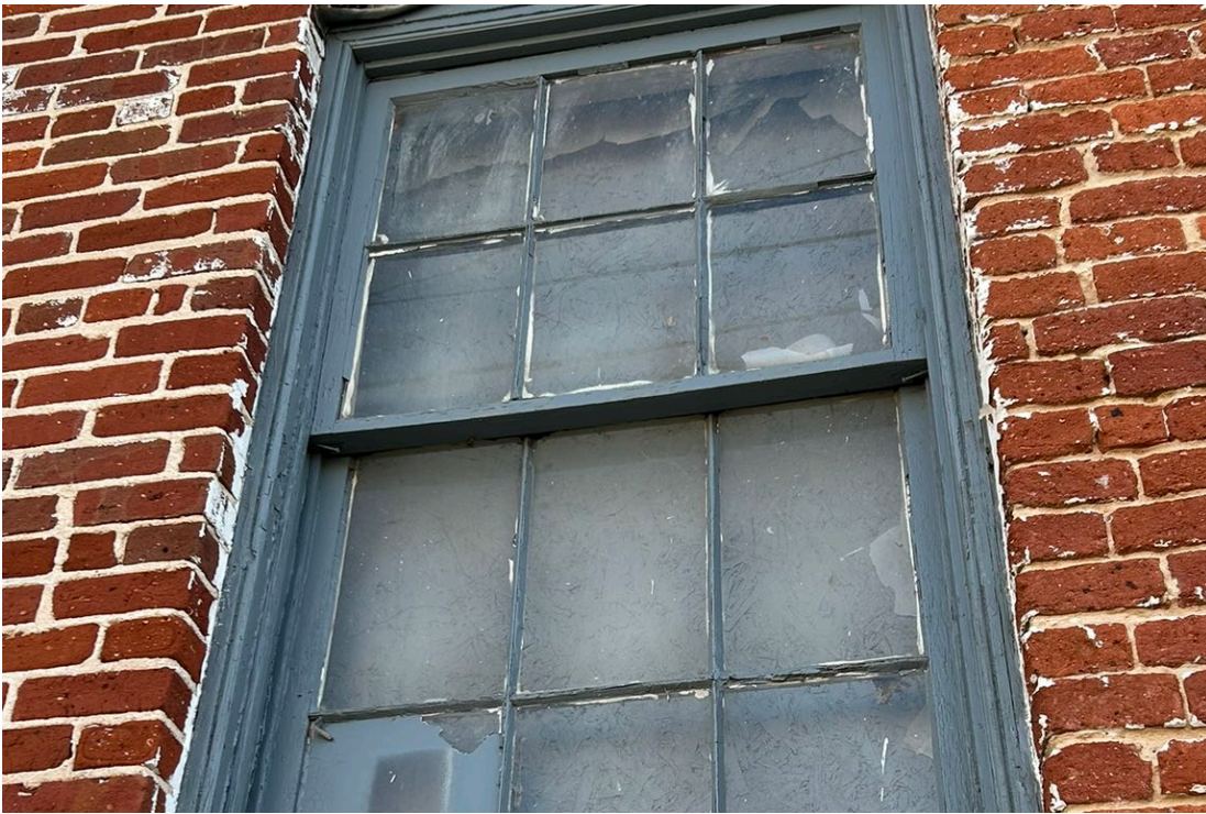
Photo 4I: Windows, Section D conditions: deteriorated rails and stiles, muntins, and glazing, broken panes
