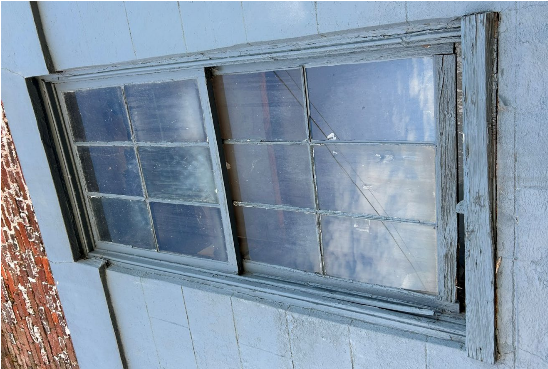
Photo 4E: Windows, Section A typical conditions: deteriorated rails and stiles, muntins, and glazing
