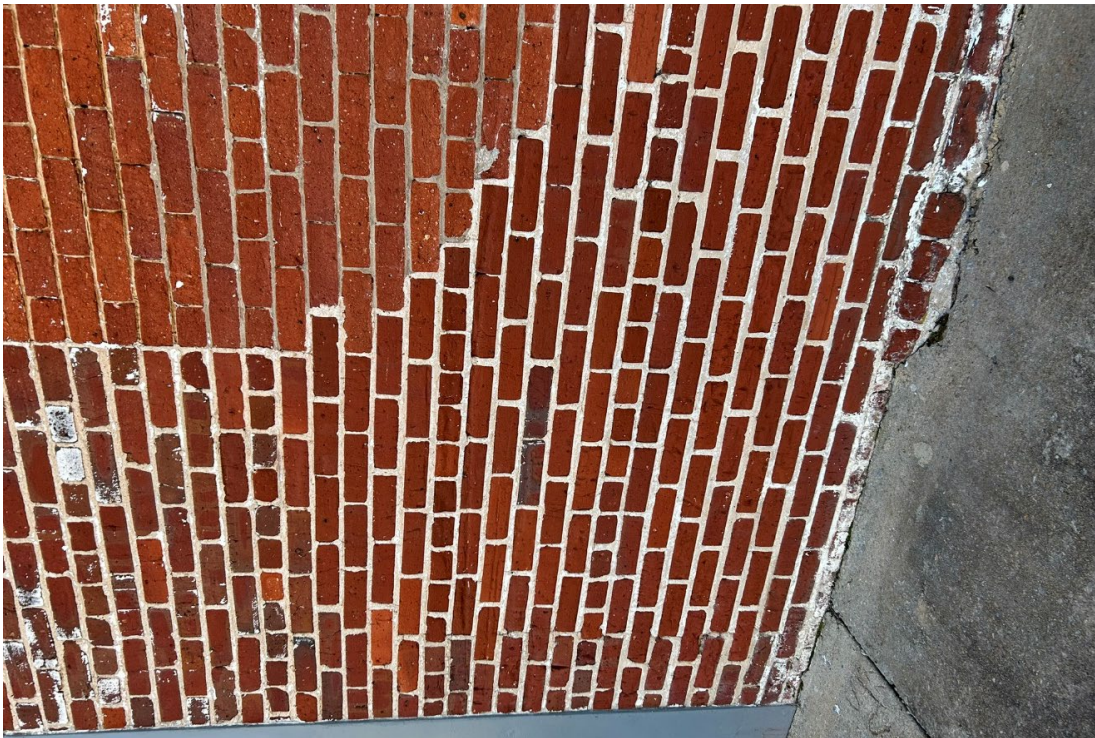
Photo 4C: Exterior Brick Walls, detail of typical brick wall condition after poorly executed paint removal
